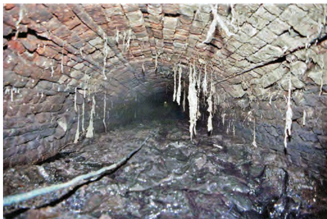
In 1991 the Hollingwood Common Tunnel was found to be heavily silted and soon became impassable.
